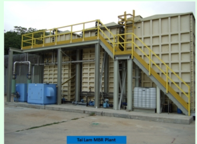
Tai Lam MBR Plant
