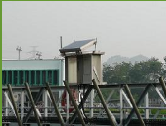
Use of Solar Energy in Sewage Treatment Plant
