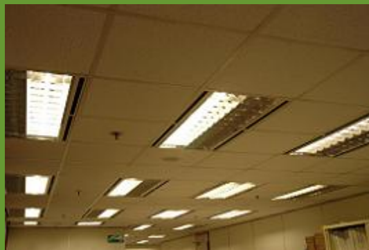
Reduced Lighting in Office
