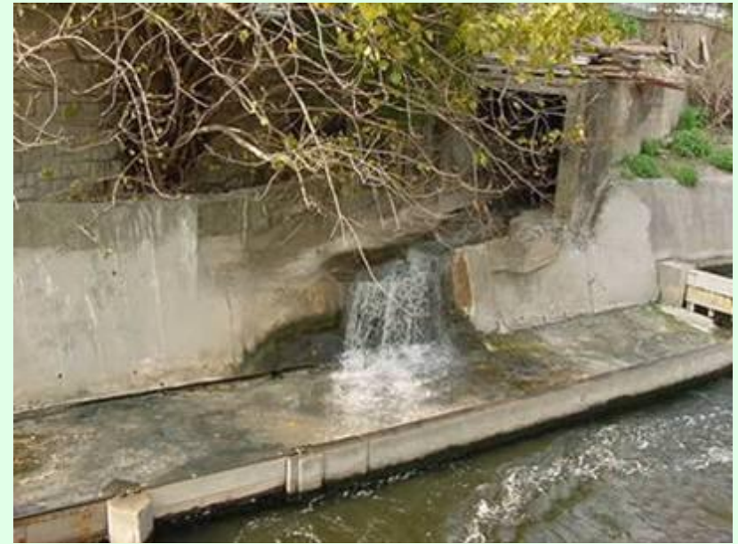
Dry weather flow interceptor at Kai Tak nullah for diverting polluted flow to foul sewer.
