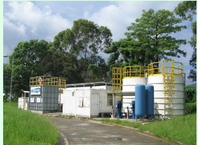
Pilot Plant for Effluent Reuse in Shek Wu Hui
