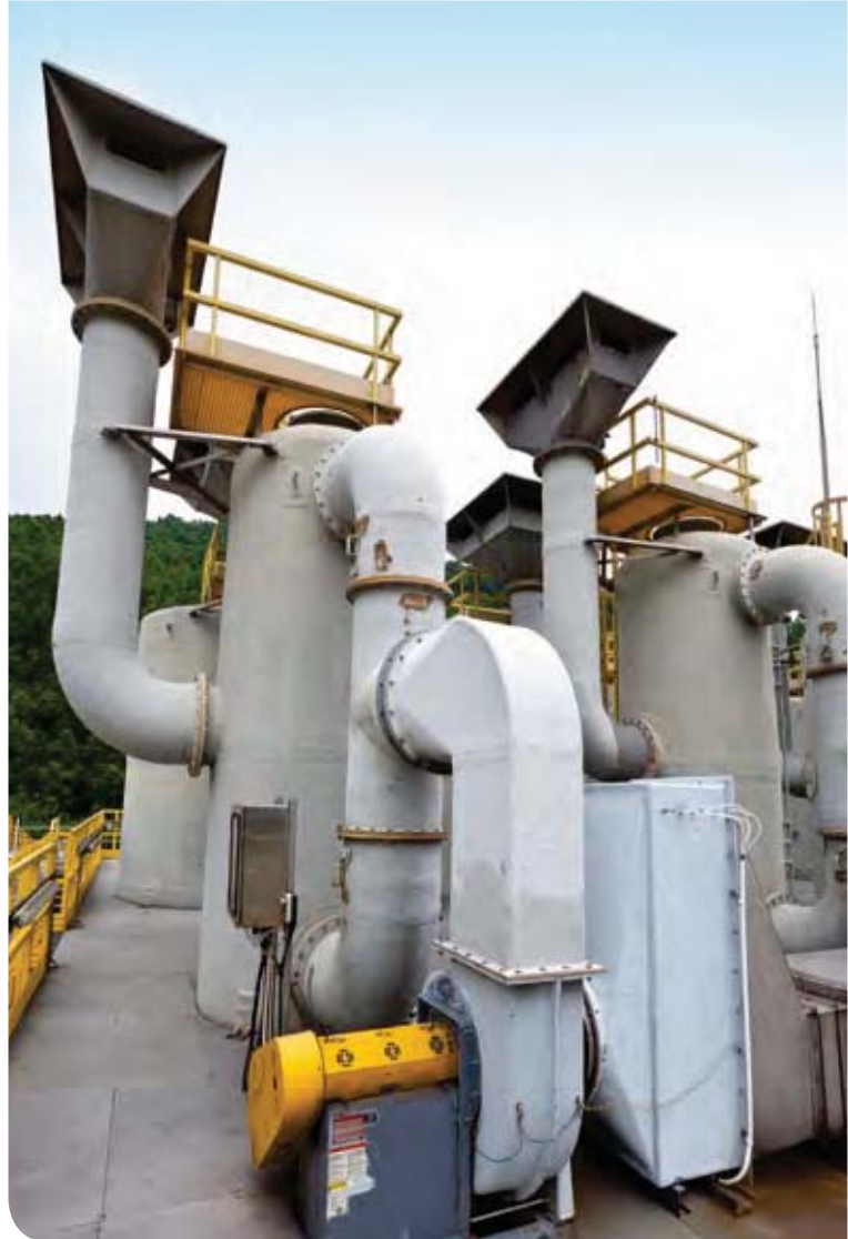
Deodorization unit at Tseung Kwan O Preliminary Sewage Treatment Works
