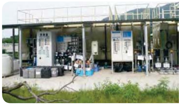
Membrane Bioreactor and Reverse Osmosis Plant at Siu Ho Wan STW
