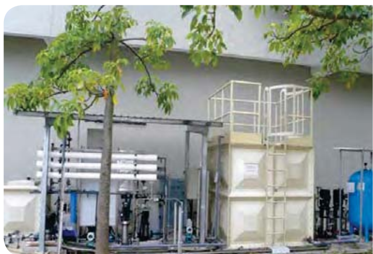
Reverse Osmosis Plant at Yuen Long STW
