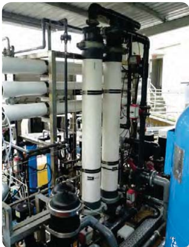
Ultra-filtration Plant at Sai Kung STW
