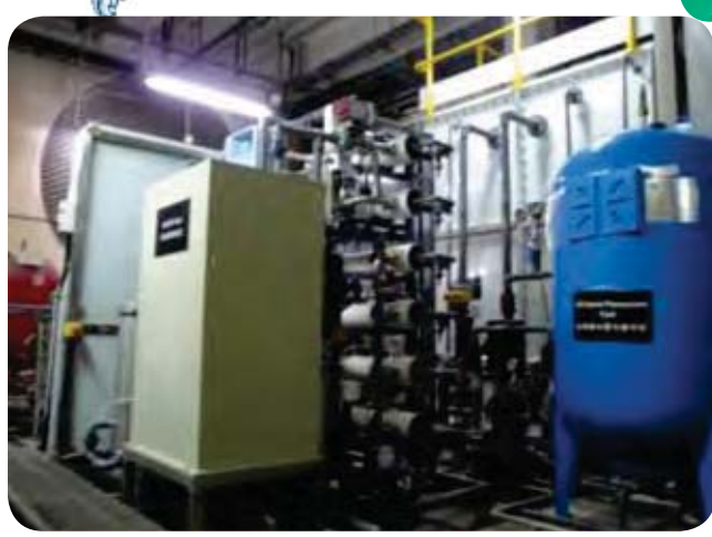
Reverse Osmosis Plant at Stanley STW
