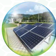
廈村污水泵房的太陽能光伏板 PV panels at Ha Tsuen Sewage Pumping Station
