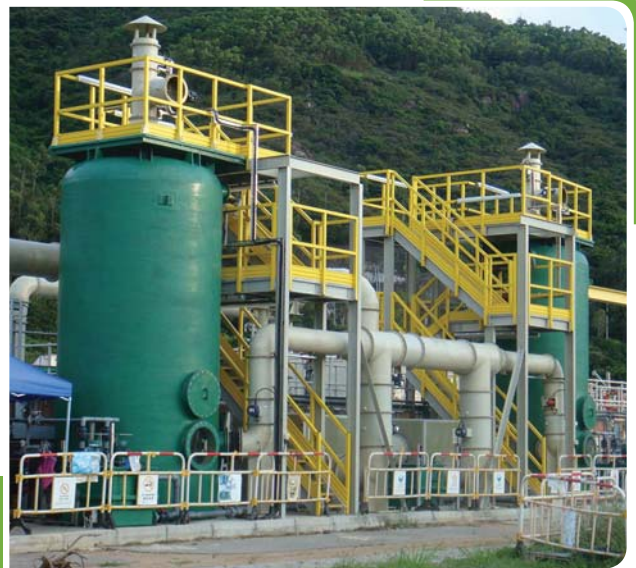
生物滴濾塔除味裝置 Biotrickling Filters
