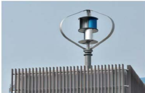
Small scale wind turbine
