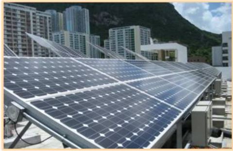
Mono-crystalline PV panels
