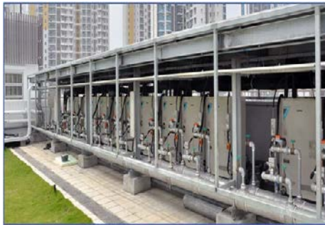
Water cooled VRV system
