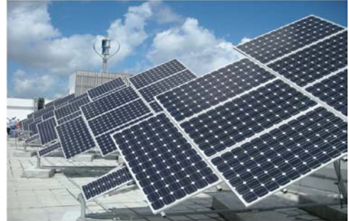
Mono-crystalline PV panels with sun tracking
