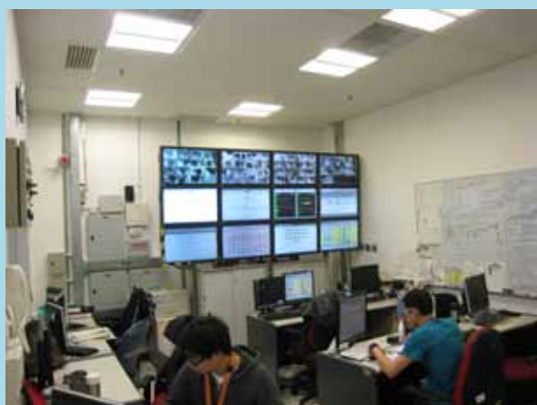
Operation room at Kowloon Bay Data Centre
