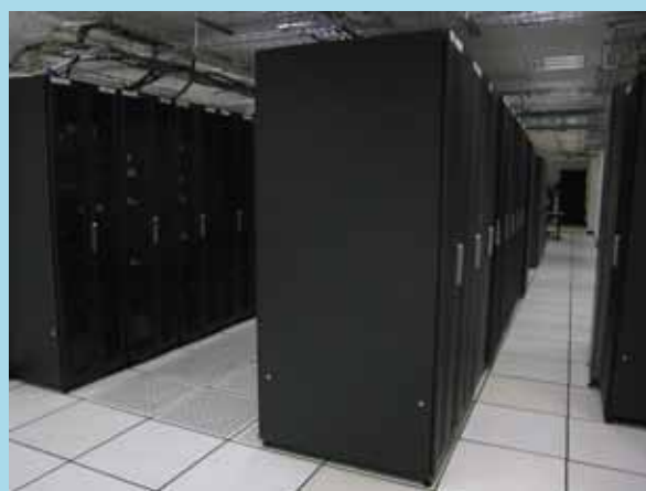
Server racks arranged in "hot" and "cold" aisles configuration
