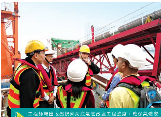
▶ 工程師親臨地盤視察海底氣管改道工程進度，確保氣體安全，以配合啟德郵輪碼頭發展。 Engineers carrying out on-site gas safety inspection of the submarine gas pipeline diversion works for the development of the Kai Tak Cruise Terminal.
