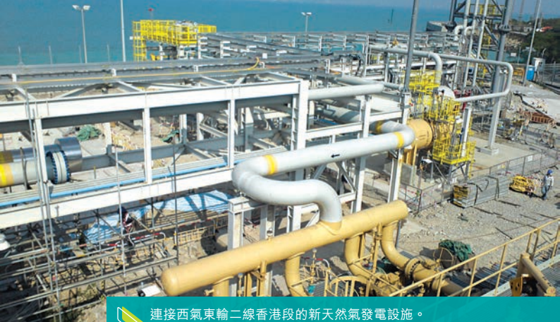
▶ 連接西氣東輸二線香港段的新天然氣發電設施。 New natural gas facilities for power generation connecting to the Hong Kong section of the Second West-East Gas Pipeline.
