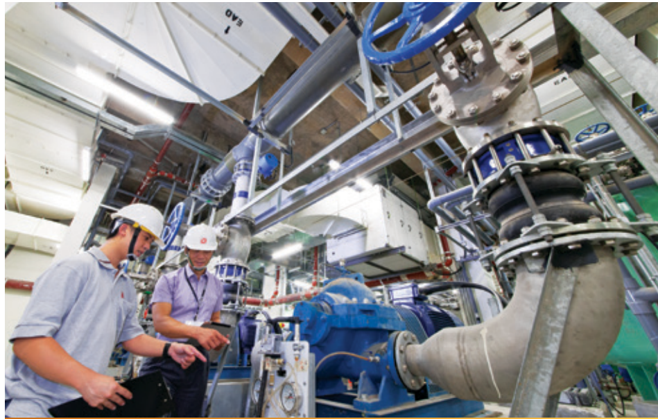
我們的專業人員為新屯門西北游泳池的過濾系統進行定期檢查。 Our professional staff is conducting regular inspection of the filtration system at the new Tuen Mun North West Swimming Pool.
