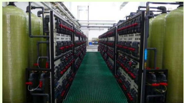
Ion exchange system employed in a plastic product manufacturing factory to recycle rinsing water.
