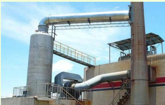
Renovated boiler flue gas in textile factory with enhanced effectiveness.
