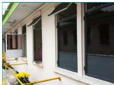
Solar film installation in one of the energy improvement works under the Energy Conservation Projects for NGOs Scheme.
