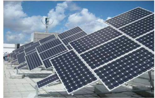
Mono-crystalline PV panels with sun tracking
