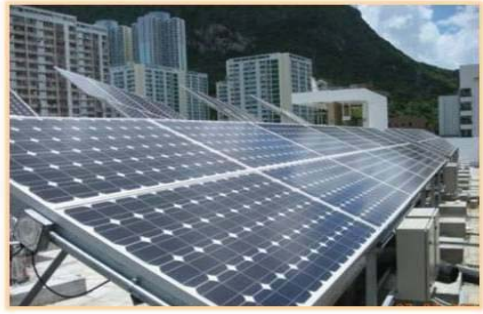
Mono-crystalline PV panels
