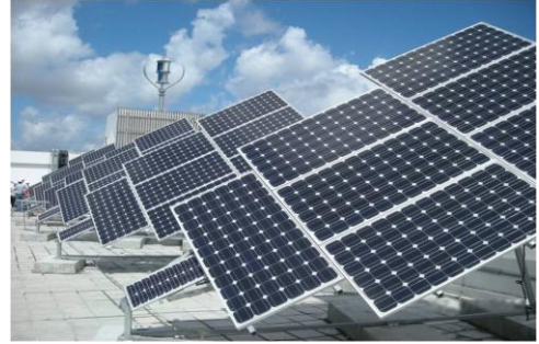
Mono-crystalline PV panels with sun tracking
