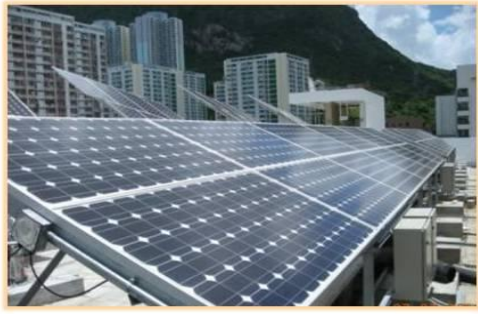
Mono-crystalline PV panels
