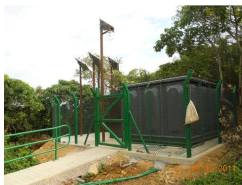
Provision of solar light system for a water tank at Chau Mei, Sai Kung North, Tai Po
