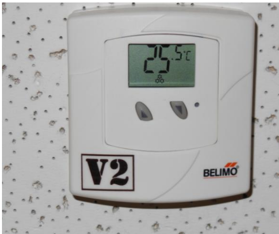
Maintaining air-conditioned room temperature at 25.5°C
