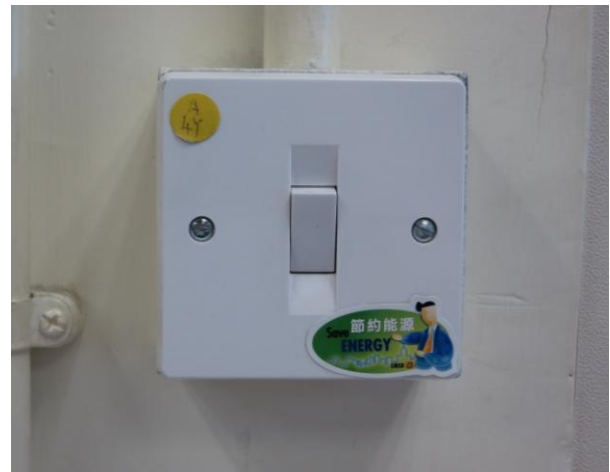
Affixing "Save Energy" stickers near the switches
