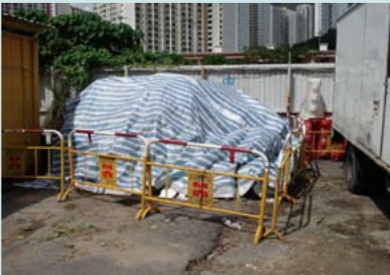
Dusty material covered up
