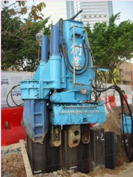
Silent piler was used for driving sheetpiles in front of Kwai Tsing Theatre
