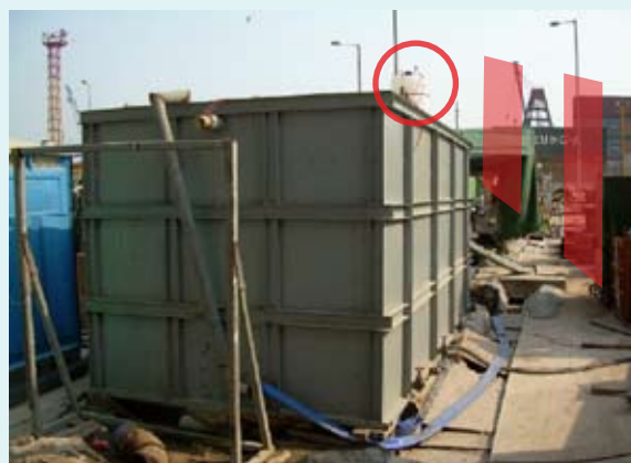
Sedimentation tank with flocculant dosing
