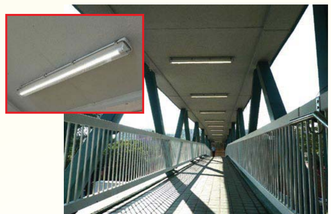
LED Light Tubes for Footbridge
