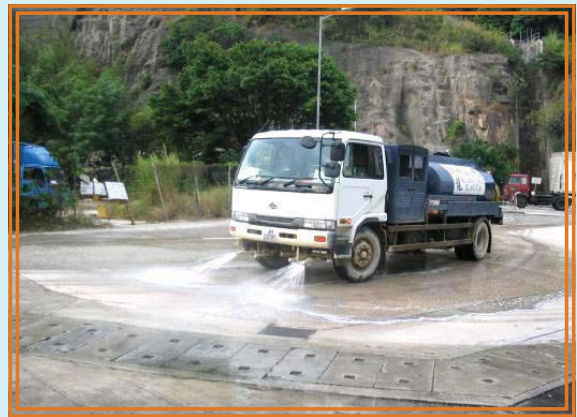
Use of water lorry equipped with spray nozzles to suppress dust generation
