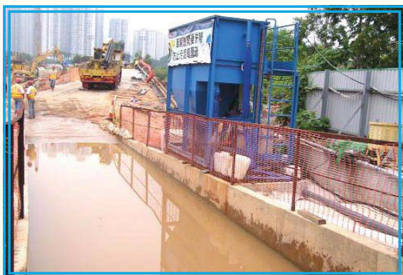
On-site wastewater treatment facility
