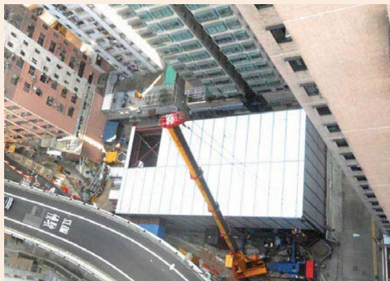
Noise Enclosure at Hill Road
