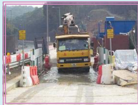
Wheel washing basin
