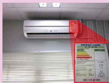
Air Conditioners for site office have Energy Efficiency Grade 1 under the Energy Efficiency Labelling Scheme
