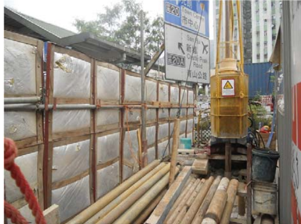
Movable noise barrier
