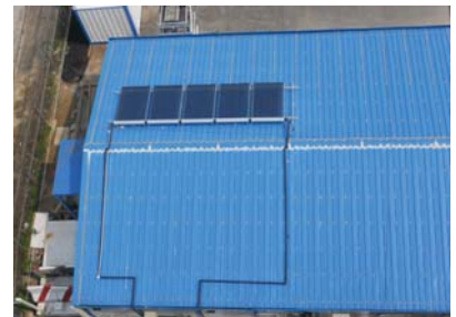
Solar panels for water heater in site office
