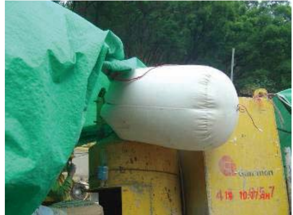
Exhaust air dust bag for grouting station
