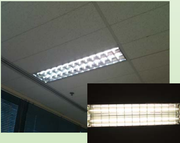
T5 fluorescent lighting
