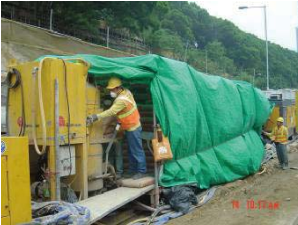
Dust enclosure for grouting station
