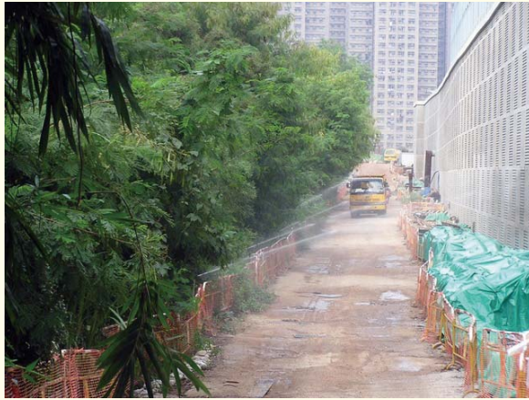
Automated water sprinkler at haul road
