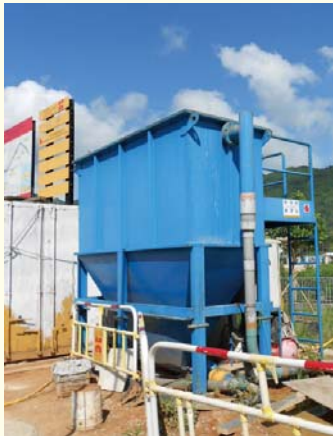
On-site wastewater treatment facility
