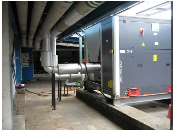
New Energy Saving Chillers for A/C Units
