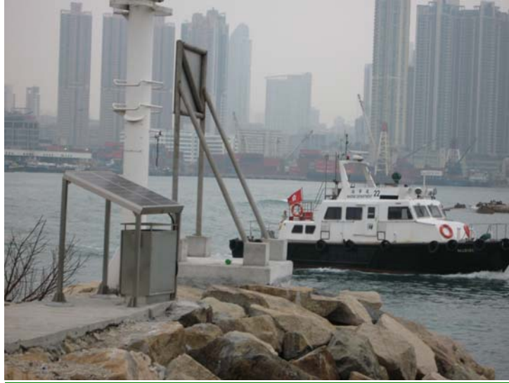
Photovoltaic Motion Detection Sensor to Monitor GD's Breakwater Security
