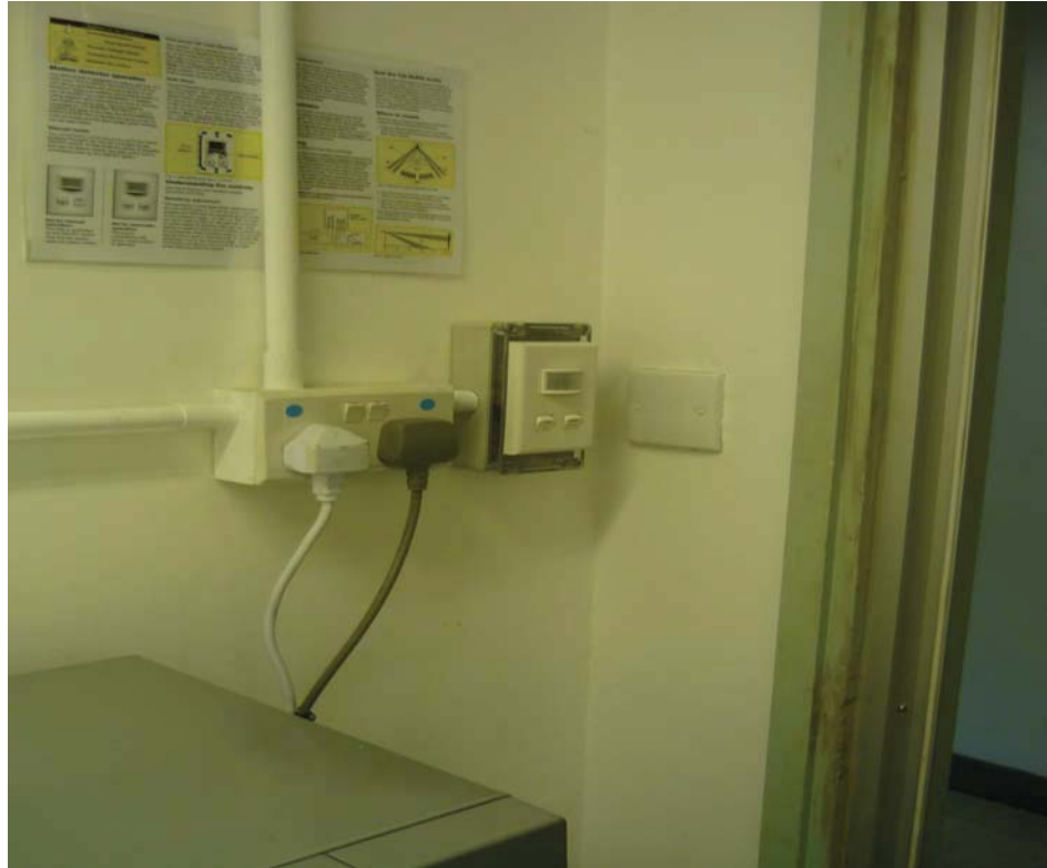
Proximity switch in the Administration Building pantry
