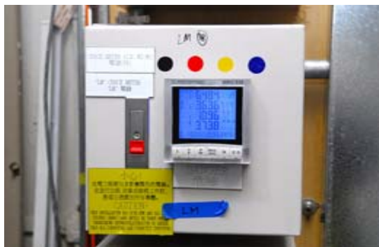
Meters are installed to monitor the electricity
