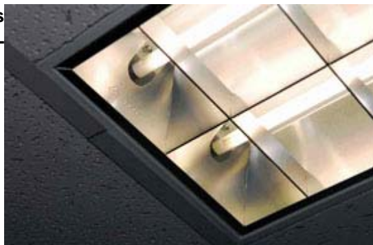
Thin fluorescent light tubes (T5) are used to reduce power consumption.
