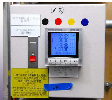
Meters are installed to monitor the electricity consumption of the floor.
