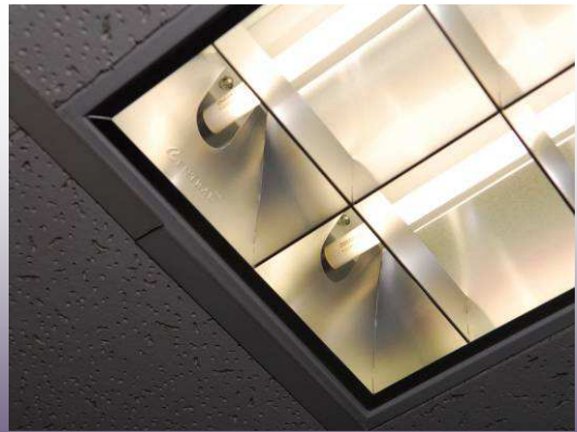
Thin fluorescent light tubes (T5) are used to reduce power consumption.
