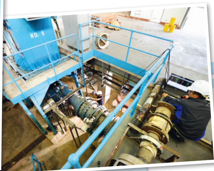
密切監察抽水泵組的效率。 Closely monitoring the efficiency of pumpsets.
