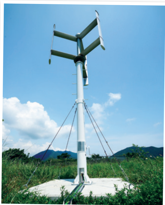
設於紅山濾水廠的直立風力發電設施。 A vertical wind turbine at Red Hill Water Treatment Works.
