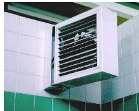
Solar Power Driven Ventilation Fan installed in the public toilet at Victoria Park Proper
