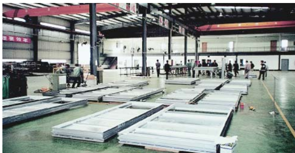
Prefabrication of the unitized curtain walls and stone faced precast walls off-site.
