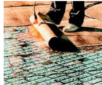
"Foamglas" made of recycled glass with low embodied energy is used as insulation materials on roof.
