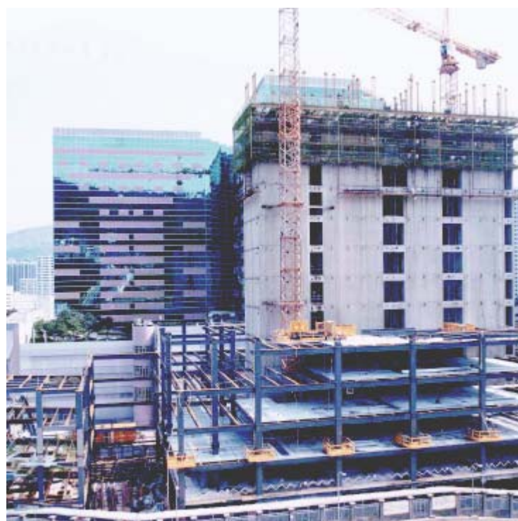
Construction of the hybrid Structure – concrete core walls and structural steel frame.
