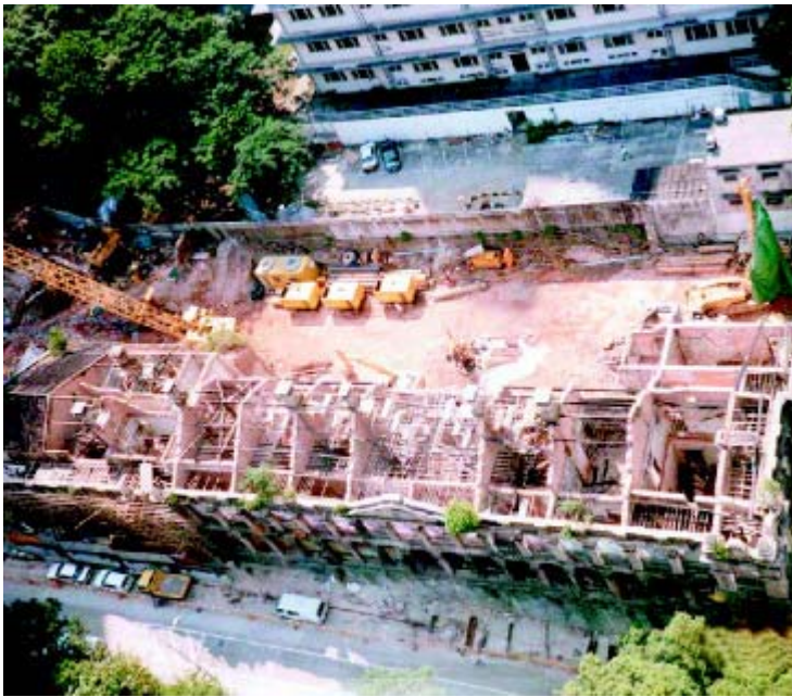
The old mental hospital being demolished for the construction of a new community centre and a singleton hostel while preserving the old façade.
