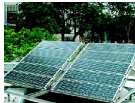
Photovoltaic Panels installed on the roof of public toilet for the generation of Solar Power
