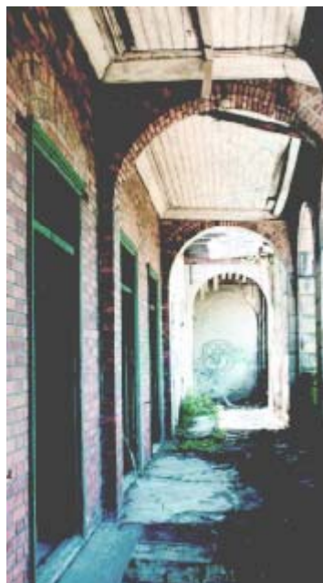
The dilapidated verandah of the Old Mental hospital.
