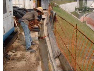
Clearing site drainage system to ensure free flow of water - an anti-mosquito measure
