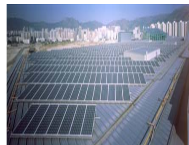
PV panels at EMSD Headquarter roof top
