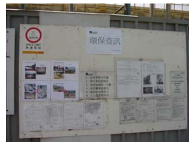
Environmental bulletin board for contractor's site staff
