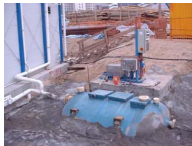
EPD - approved biological sewage treatment plant was deployed and checked regularly
