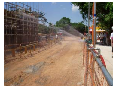
Automatic water spraying system for dust control
