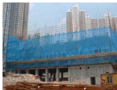
Perimeter screen was provided higher than working level for better dust screening
