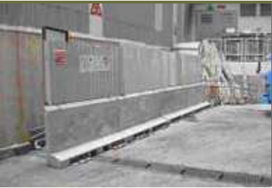
Precast concrete road paving and reusable precast concrete hoarding were used extensively
