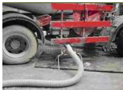
Vehicle exhaust gases filtration system
