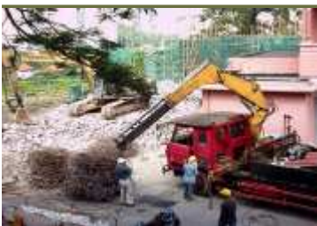
Waste materials generated from demolition of an existing building were sorted for recycling
