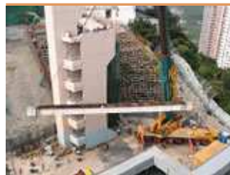
Lifting arrangement to take down a beam of large span in a demolition project
