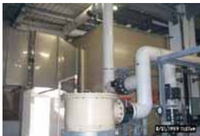
Water scrubber to reduce odours
