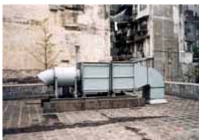
Existing carbon filtration system in RCP
