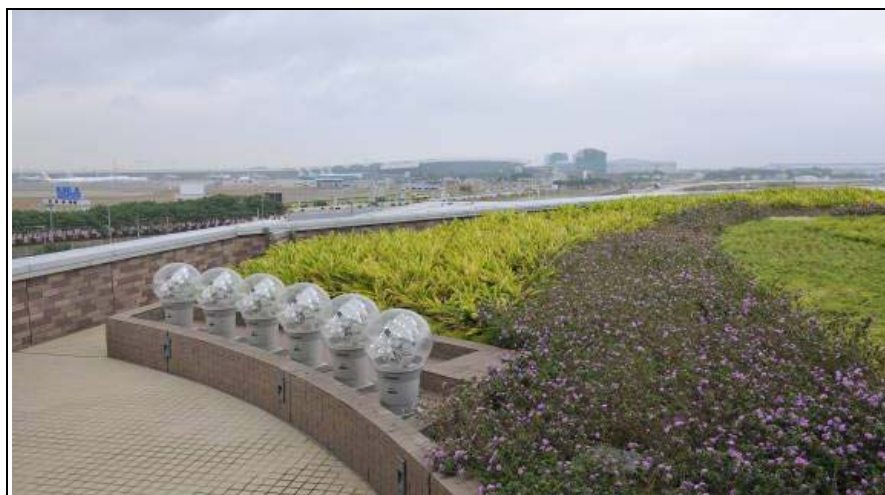
Figure 10: Solar Lighting Collectors with Fibre Optic Solar Tracking at the CAD Headquarters
