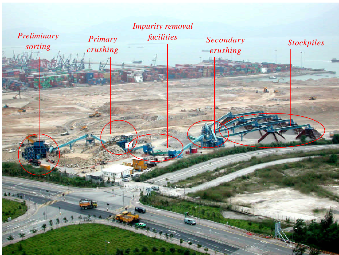
Pilot C&D materials recycling facility in Tuen Mun Area 38
