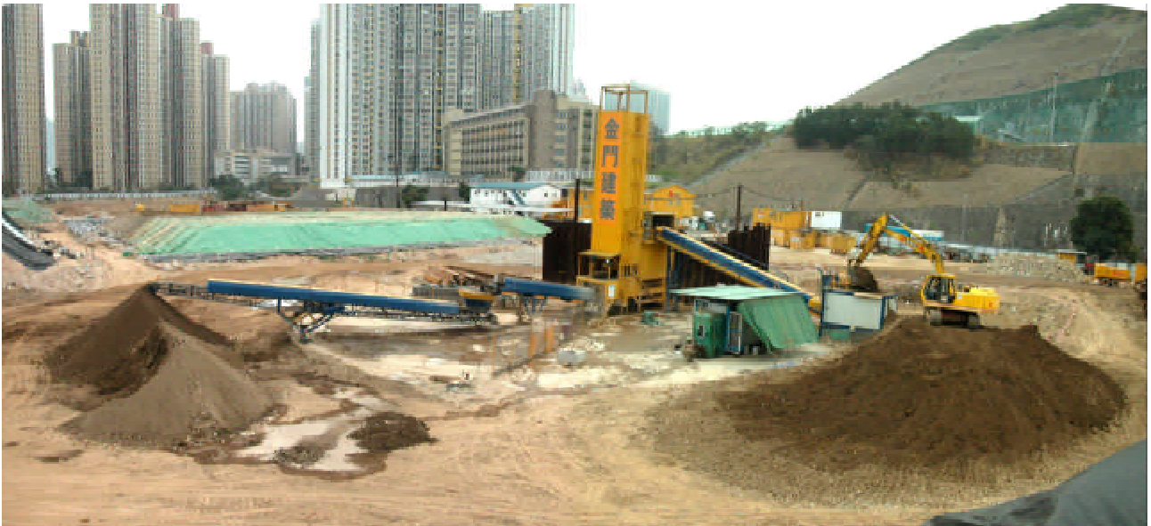
A general view of the cement solidification plant
