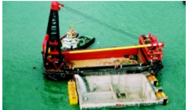
採用預製件方法建造海水泵房以減少建築廢料 Precasting Seawater Pumping Station to reduce Construction Waste
