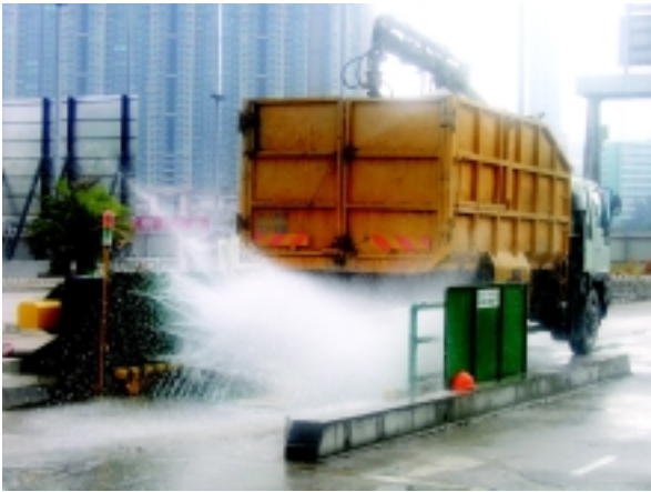
車輛離開前先在洗車處清洗車輪 Cleaning a Vehicle at the Wheel Washing Facility
