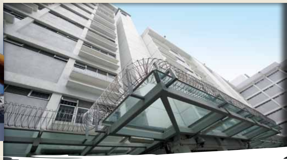
騰空的荔枝角懲教所正改建為荔枝角收押所一部分。 Works are underway to amalgamate the vacated Lai Chi Kok Correctional Institution into Lai Chi Kok Reception Centre.
