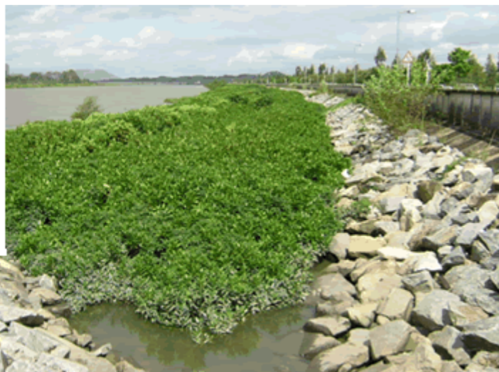
Mangrove created along the bank of Kam Tin River to provide compatibility and integration with the environment
