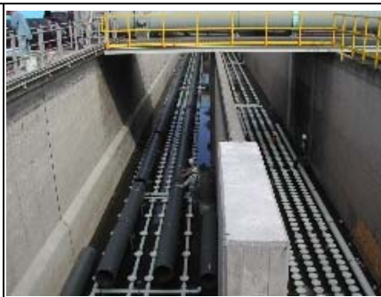
Shatin STW aeration tank
