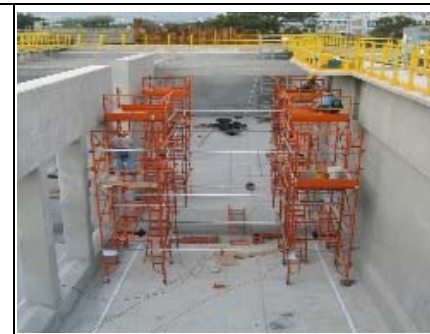
Shatin STW sedimentation tank
