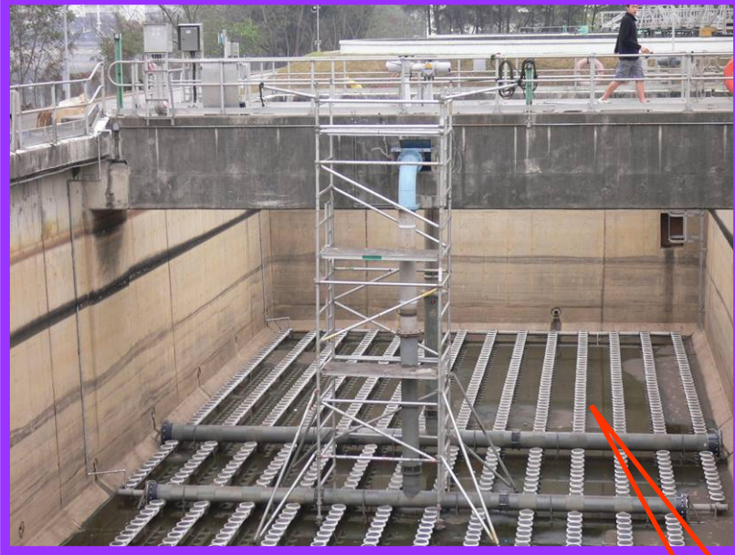
Membrane type fine bubble air diffusers, which are more energy efficient, have been adopted at Yuen Long Sewage Treatment Works.
