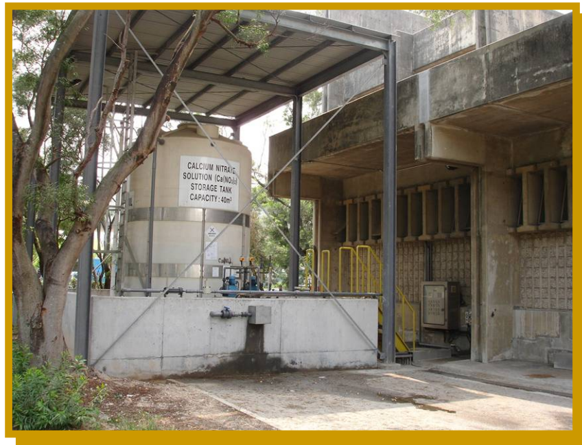
A calcium nitrate dosing system at Shatin Main Sewage Pumping Station.
