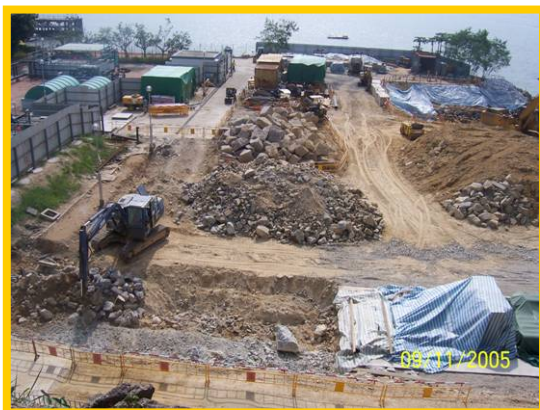
A Best Construction Sites Housekeeping Award was awarded to the contractor who managed the upgrading work at the Peng Chau STW. Site staff properly sorted and stockpiled excavated materials, which will be re-used in future backfilling work.
