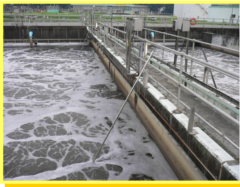
Power requirements at Yuen Long Sewage Treatment Works have been reduced by replacing 400 kW air blowers with 200 kW air blowers and installing an automatic dissolved oxygen control for aeration tanks.
