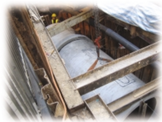
A 1500 mm diameter concrete drain pipe was being laid along Queen's road central to address the flooding problem in Sheung Wan
