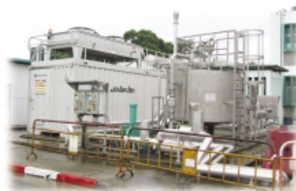
Combined Heat and Power Generator at Shek Wu Hui Sewage Treatment Works
