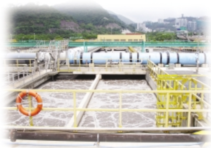
More efficient aeration system adopted at Shatin Sewage Treatment Works
