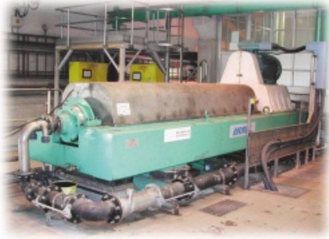
A new type of centrifuge with energy-saving features at Stonecutters Island Sewage Treatment Works
