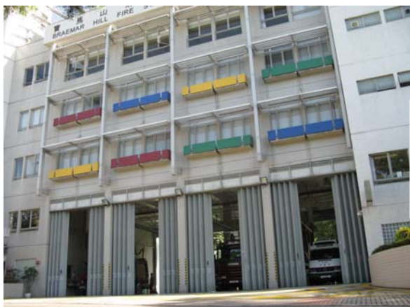
Folding gates at Fire Station installed with noise mitigation measure
