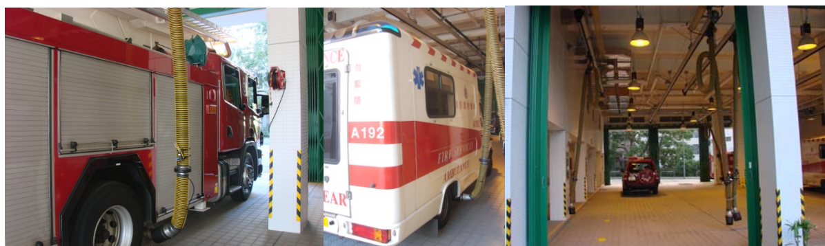
九龍塘消防局暨救護站的汽車排氣設備 Vehicle Exhaust System at Kowloon Tong Fire Station cum Ambulance Depot,
