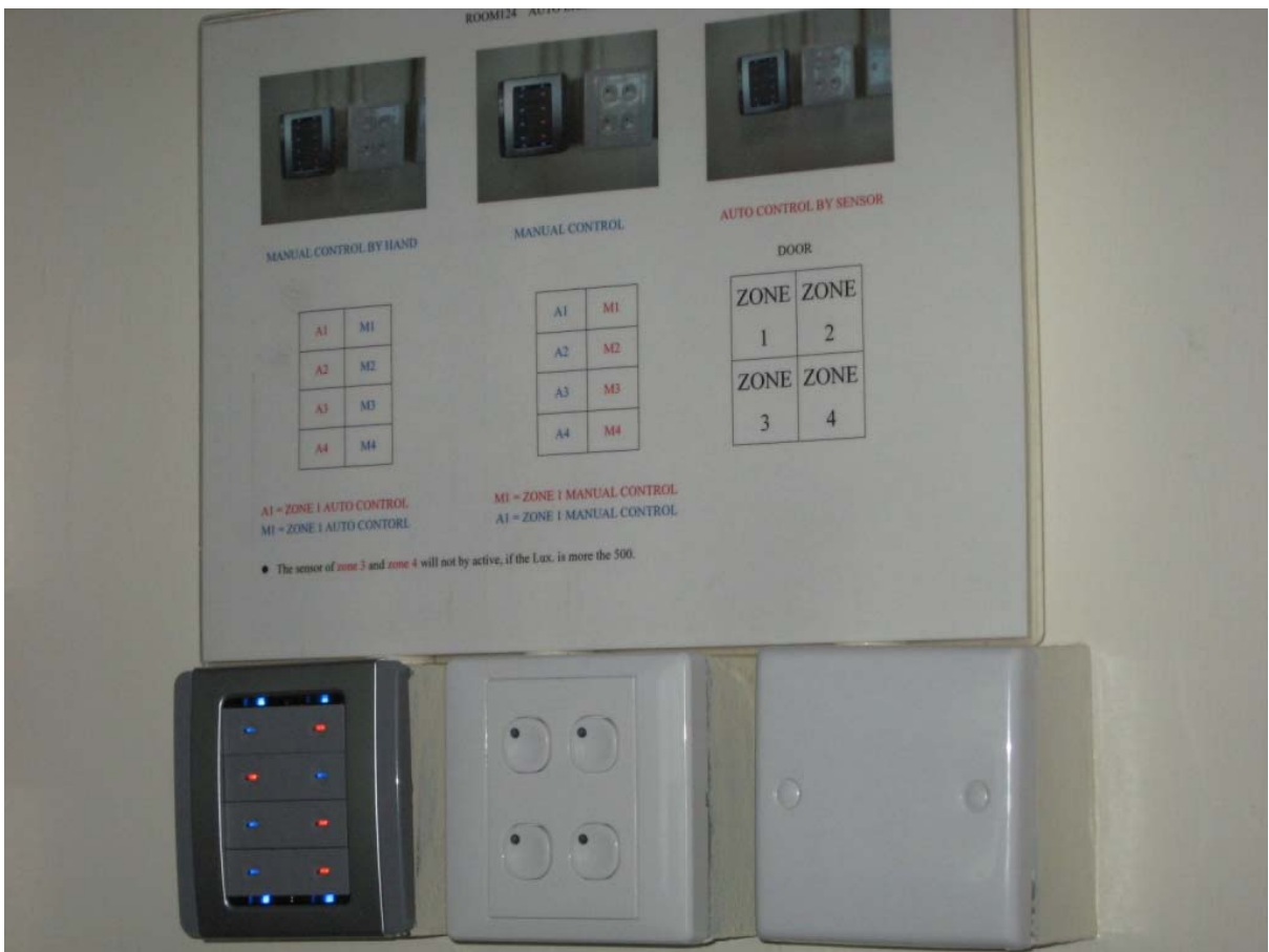
Zoned lighting and switches
