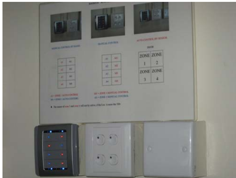
Zoned lighting and switches
