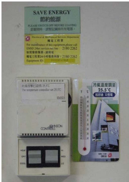
Setting room temperature at 25.5°C
