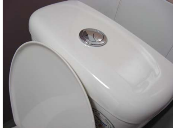
Plumbing appurtenance with water saving devices
