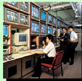
Centralized Monitoring System for Property Management
