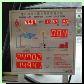
Monitoring display meter of photovoltaic panels installed in Wanchai Tower
