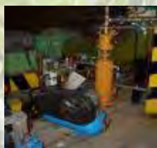
Addition of automatic tube cleaning system in Immigration Tower
