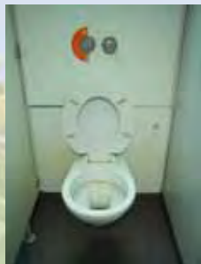
Dual flush/water saving cistern installed in some GO
