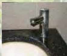
Using of sensor water faucets in GO washrooms
