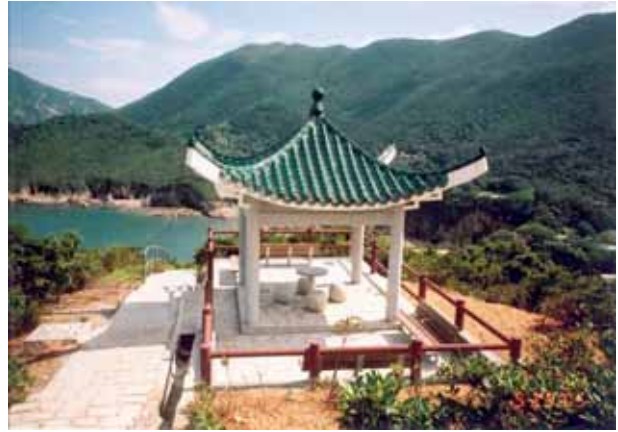
Construction of a Rain Shelter for Hikers on the Footpath Linking Pottinger Peak and Big Wave Bay Southern District
