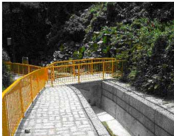
Construction of open channel at Pai Min Kok Village, Tsuen Wan District
