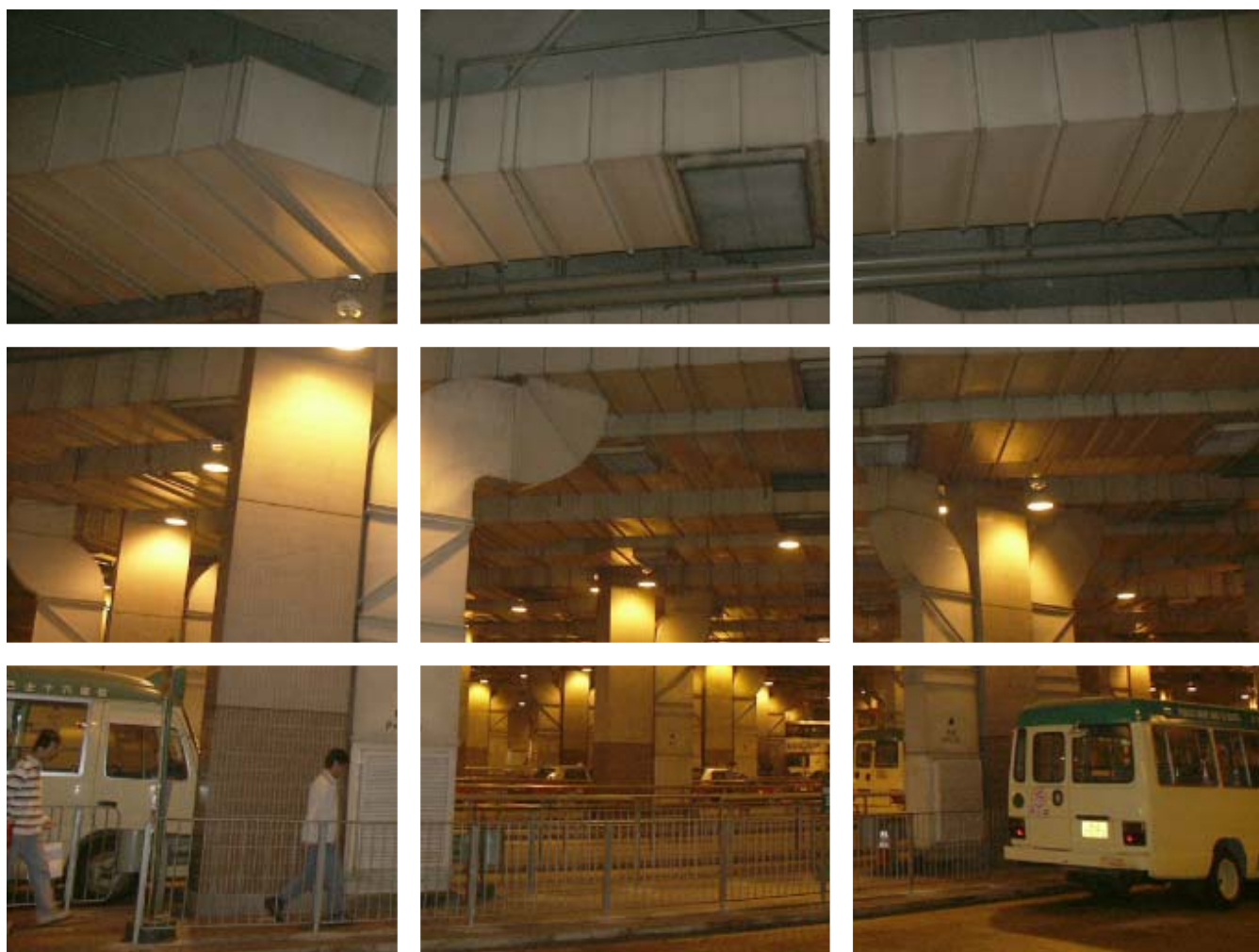
Ventilation system in PTI
