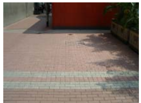
Trial of recycled aggregate block pavers at Cheung Sha Wan Road in Lai Chi Kok
