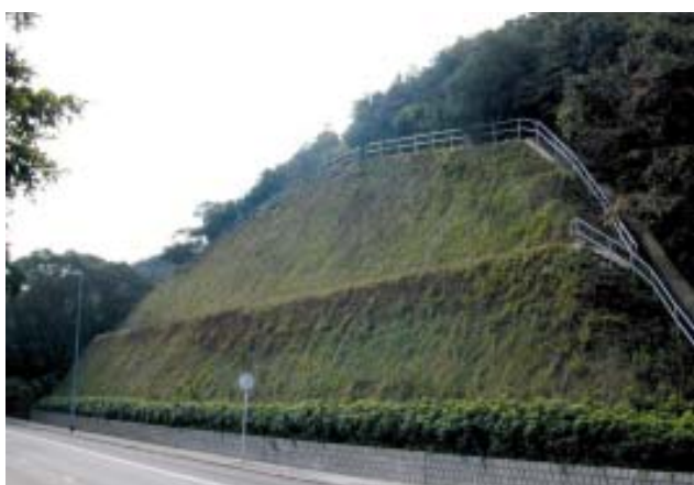
Slope at Wong Nai Chung Gap Road after greening by geo-synthetic mat system
