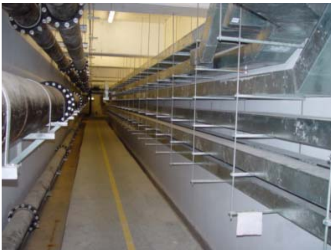
Common utility enclosure
