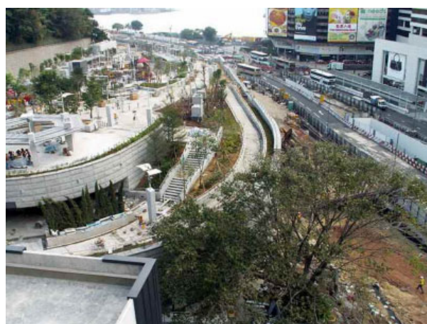
Reinstatement of Middle Road Playground by East Rail Extension from Tsim Sha Tsui to Hung Hom
