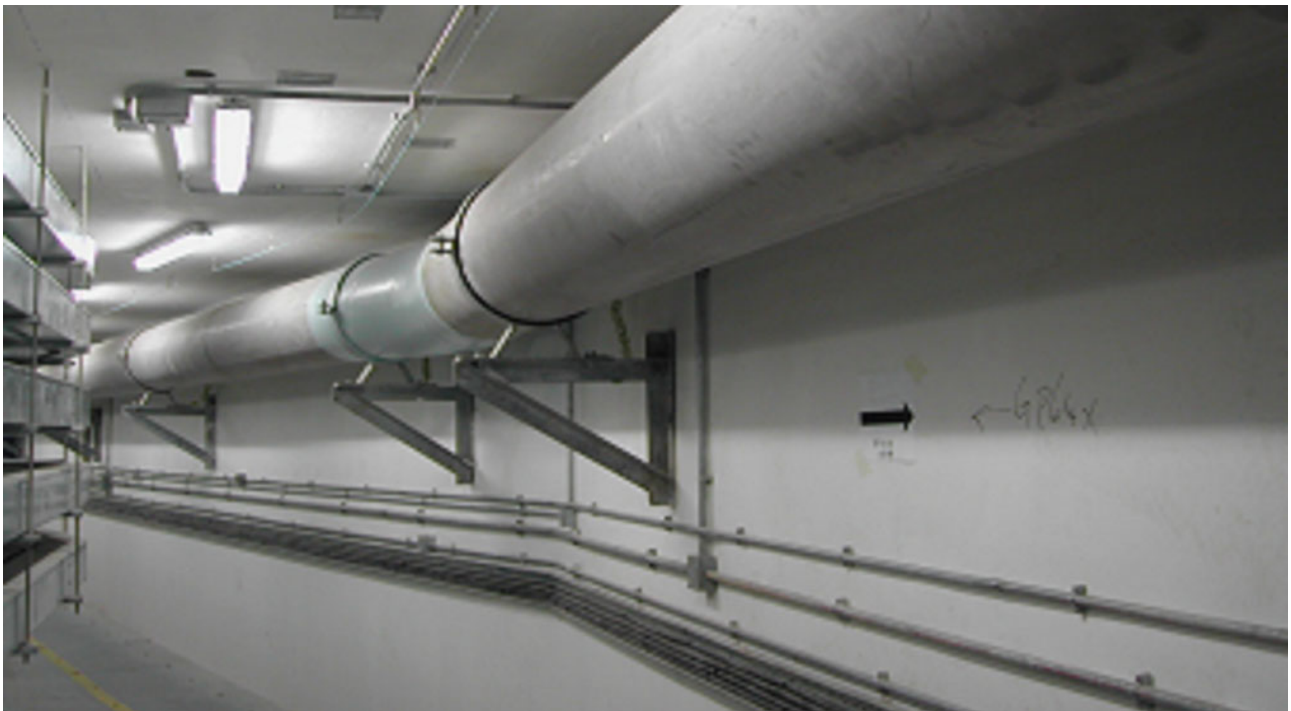
Common utility enclosure
