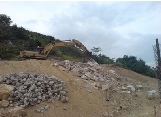
Breaking of bedrock and concrete during the formation of cut slope for reuse on site
