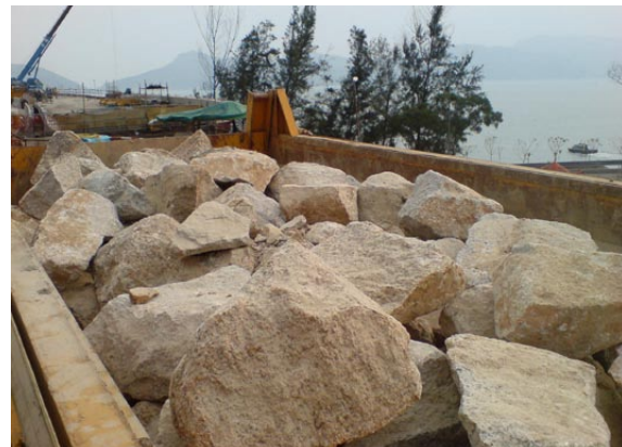
Reuse of bedrock and boulders broken on site as Grade 700 rockfill for seawall underlayer
