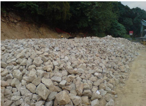
Reuse of broken rock and concrete for the construction of rock fill slope
