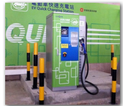
Electric vehicle charging facilities
