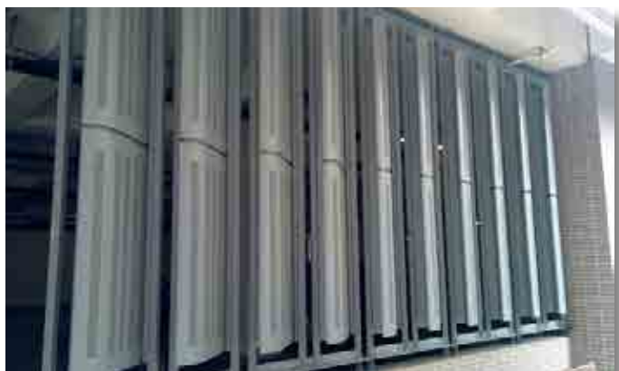
Bio-filtration units in Cheung Sha Wan Estate
