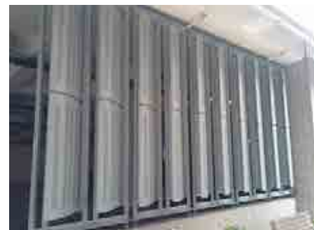
Bio-filtration units in Cheung Sha Wan Estate
