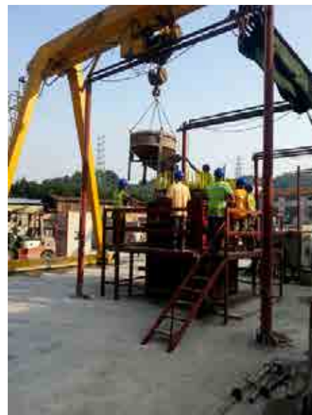
Precast manholes used in Shui Chuen O Phase 1
