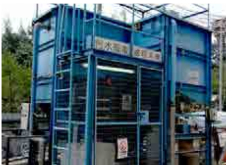
Mandatory installation of water recycling facilities
