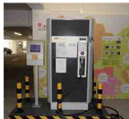
New electric vehicle charging facility in Yue Wan Estate Carpark
