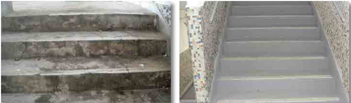
Carrying out repair and improvement works at Wah Fu (I) Estate: before repair (left) and after repair (right)
