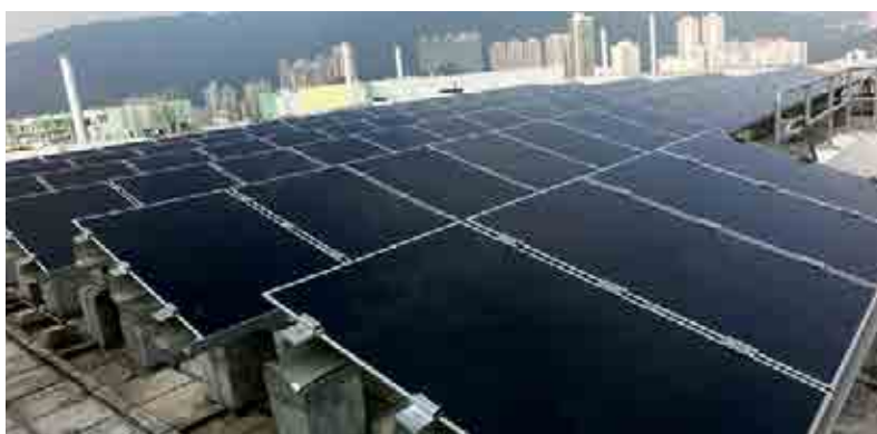
Solar panels at Kai Tak Site 1B
