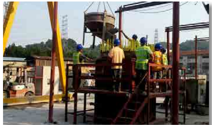
Precast manholes used in Shui Chuen O Phase 1
