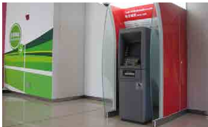
Installation of ATM in Domain
