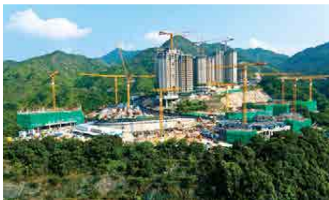
The latest 5-D BIM model has been applied to Sha Tin Area 52 Phase 1 Project
