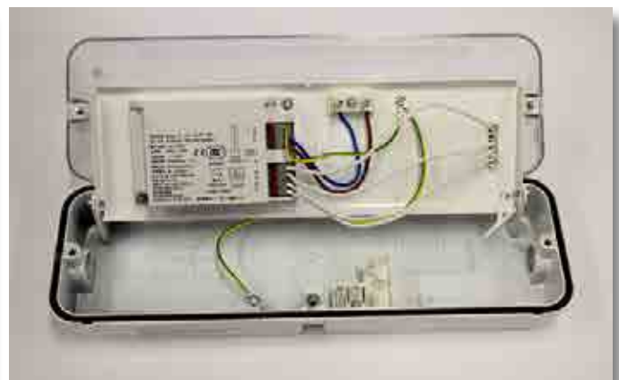
Electronic ballast bulkhead light fitting in Kwai Shing West Estate
