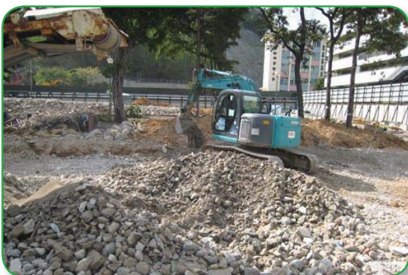
Recycled concrete used to fill up the void after the removal of a foundation.
