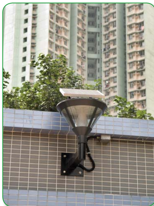
Lighting improvement in estate
