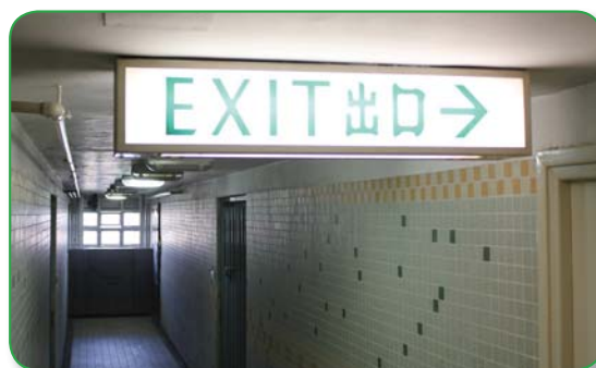
Replacement of T8 fluorescent tubes with more energy efficient T5 model in exit signs
