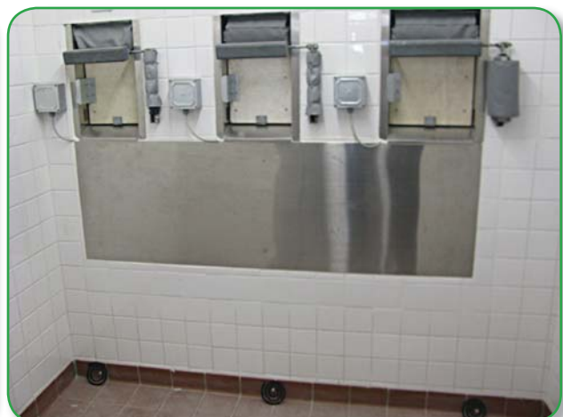
Mail-box type rubbish bins inside the refuse room in Eastern Harbour Crossing site Phase 5
