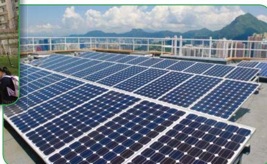
Grid-connect solar panels in Lam Tin Estate
