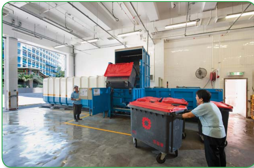
Garbage compactor system
