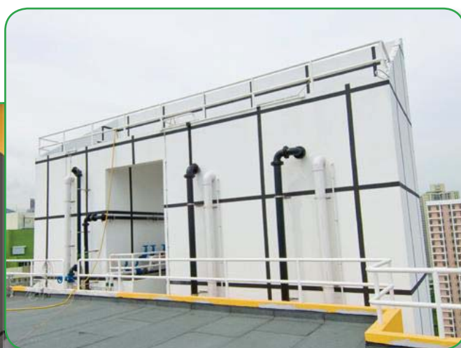
The twin tank water supply system at the roof of Yau Lai Estate in Yau Tong
