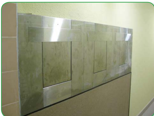
View from the corridor of the mail-box type rubbish bins in Eastern Harbour Crossing site Phase 5
