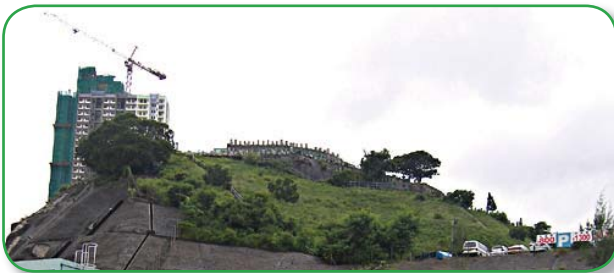
The man-made slope at the Tung Tau Cottage East Site is covered with a grass surface.
