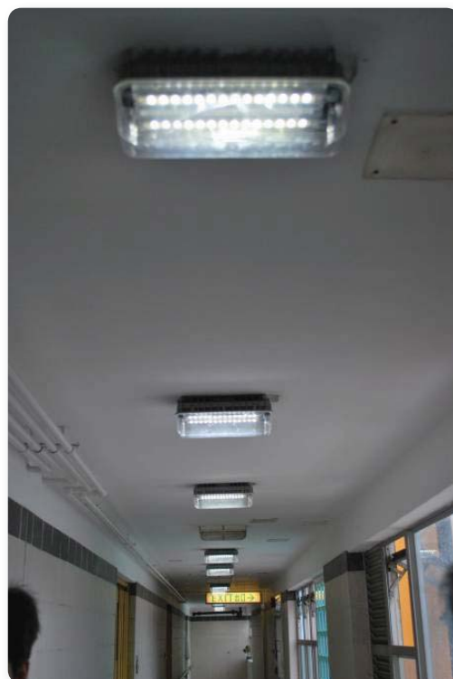
Corridor Using LED Bulkheads
