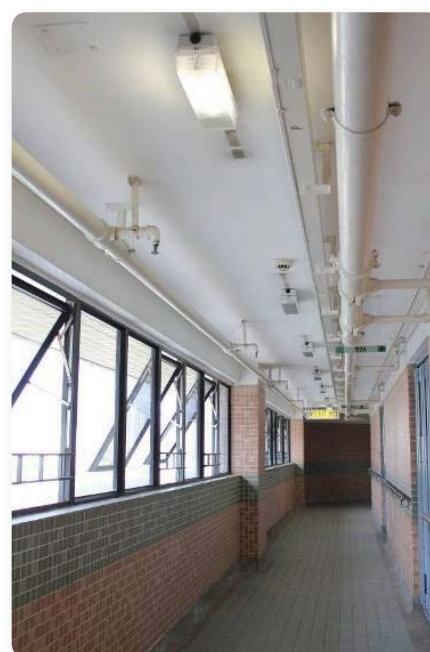
Modified Lighting Circuits in Corridor Allow Switching off Lights Selectively in Daytime in Ho Man Tin Estate
