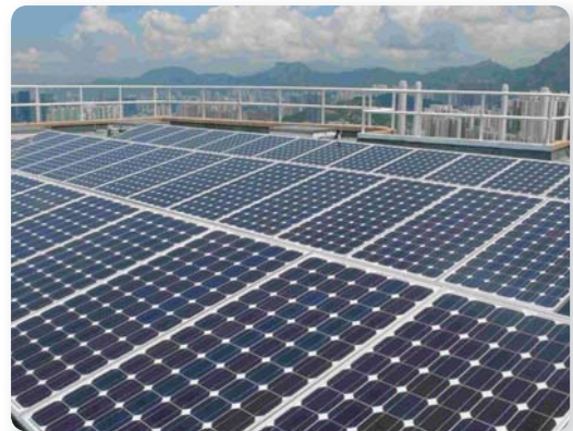
Pilot Grid-connected Photovoltaic System in Lam Tin Estate
