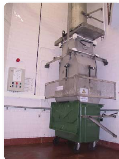
Volume Control and Storage Device of Refuse Handling System
