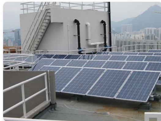
Poly-crystalline Silicon PV Modules in Eastern Harbour Crossing Site Phase 5
