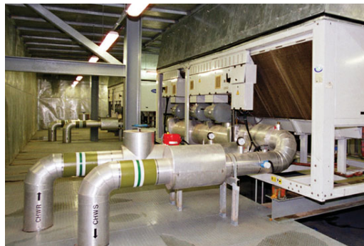
Air conditioning chillers housed in acoustic enclosure with noise silencer
