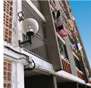
Auto lighting using photocell control system for external area in Oi Man Estate (2002)
