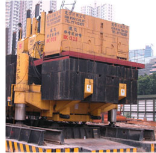
The trial of hydraulic jacking method at redevelopment of Un Chau Estate in 2002 was successful and cost effective in noise reduction
