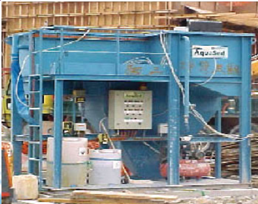
Waste water recycling system for bored piling
