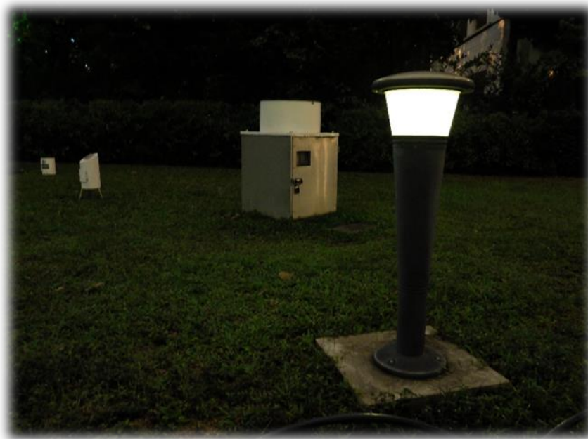
Figure 8: Solar energy lighting device
