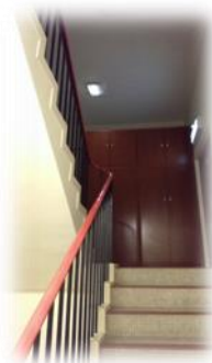
Figure 6: Lighting with motion sensors
